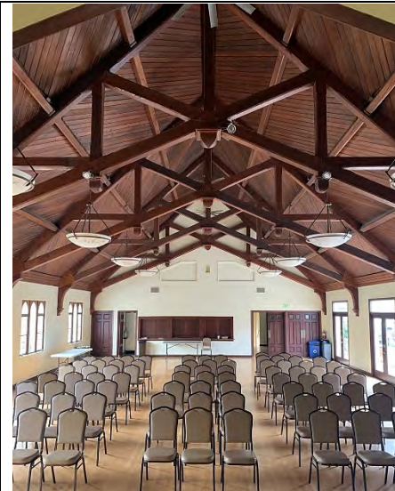
Photograph 7: Decorative scissors trusses with stained, tongue-and-groove ceiling in interior of Parish Hall. Photo by Hunter Fuentes, Historic Laguna. Not for publication.
