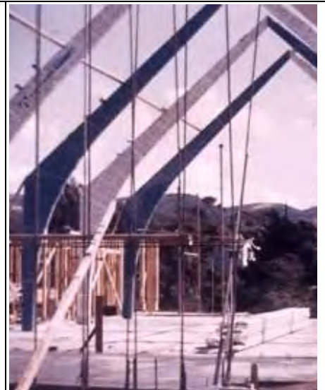
Photograph 9: Church under construction. Glulam arches were carefully wrapped during building process and positioned in the concrete foundation, unknown date. “Building Structures to Serve a Higher Purpose” Laguna Beach Independent . March 1, 2018.
